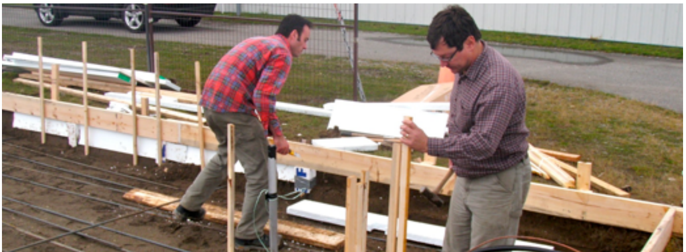
1 Don Hague marks the locations for conduits, while the contractor finishes the forming.
